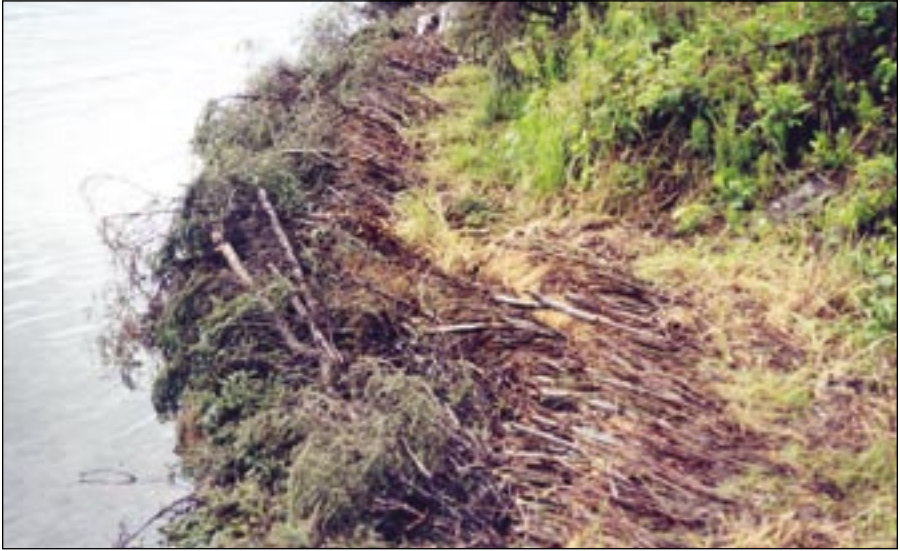
Cabled spruce trees and brush layering immediately after installation, Ciechanski Recreation Site, Kenai River
