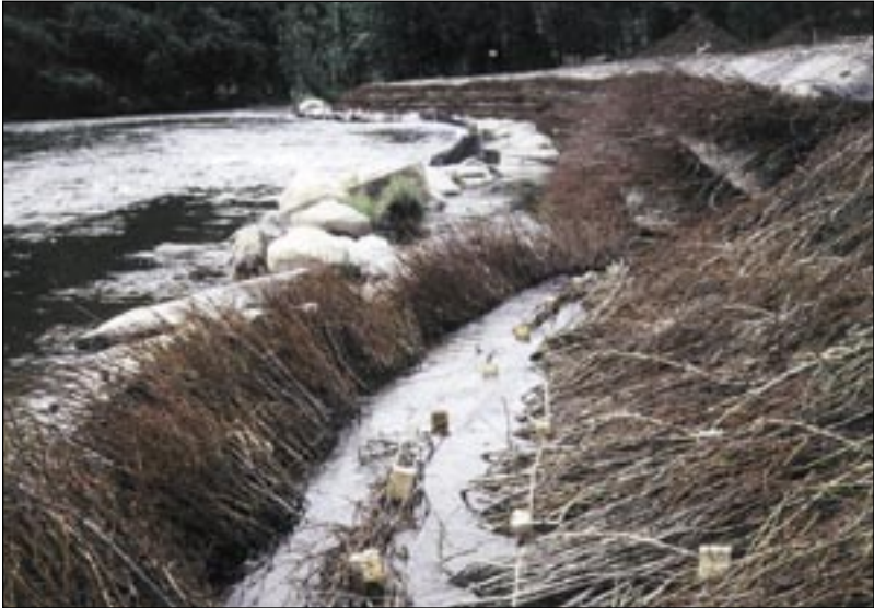
Brush mat and live siltation constructed at Deep Creek in 1994. Note bundle was used to provide a transition between the two techniques.
