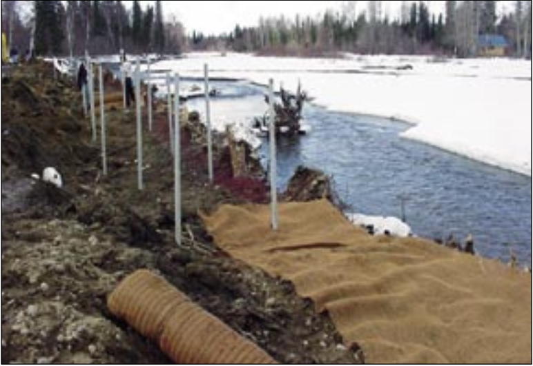
Installation of subsequent brush layering/soil wraps above root wads; the picture shows walkway supports installed. Pioneer Lodge, Willow Creek April 10-11, 2001
