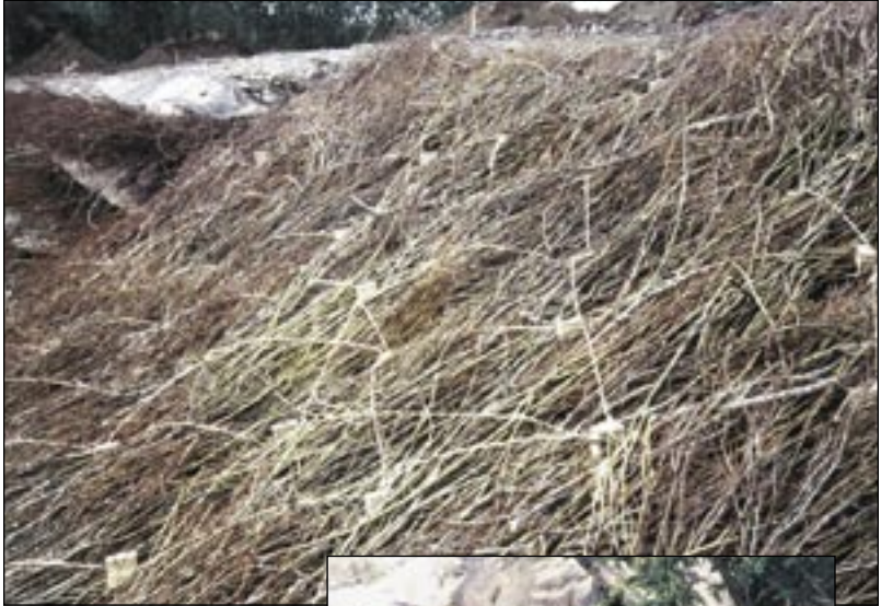
Brush mat - note the criss-cross pattern of the jute used to anchor the mat to the bank.
