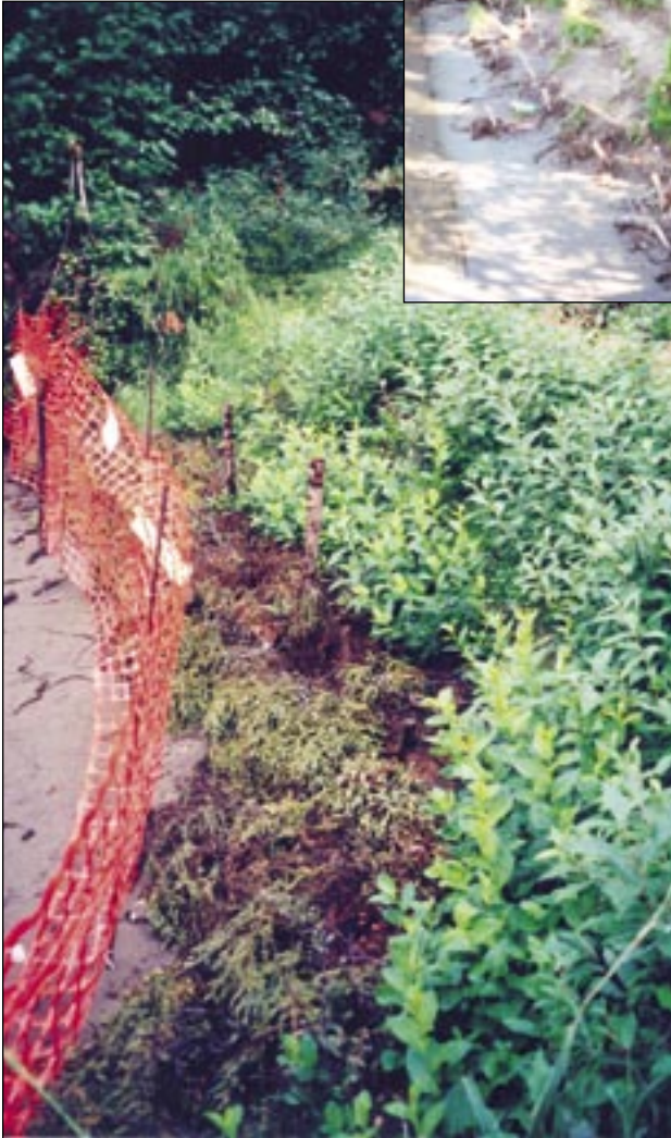
Little Susitna Recreation Site, cabled spruce trees and brush layering, three months after installation.
