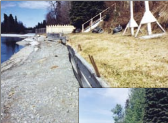
Creosote wood bulkhead prior to removal/restoration, Kenai River
